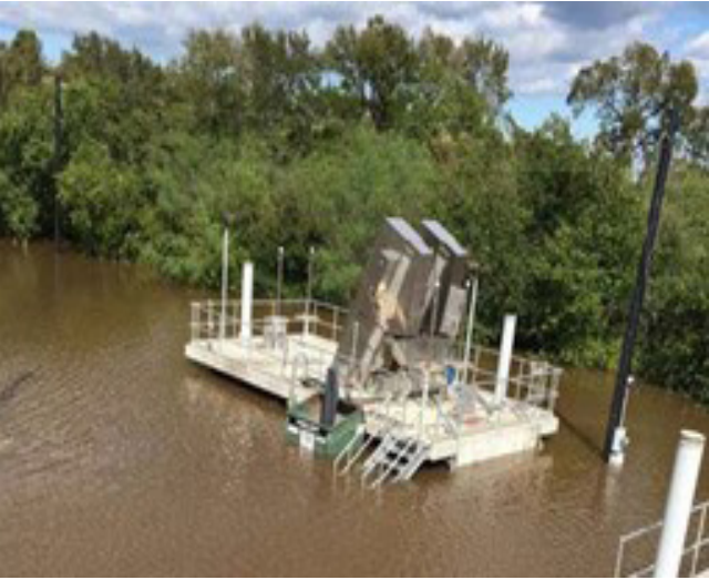
Duperon FlexRake FPFS bar screen withstands significant flooding at the City of Cuero, Texas, during Hurricane Harvey in 2017.
